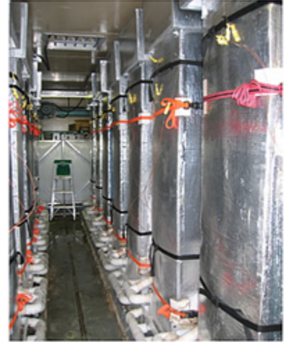
Altela ARS® 4000 water treatment towers at the demonstration site.
