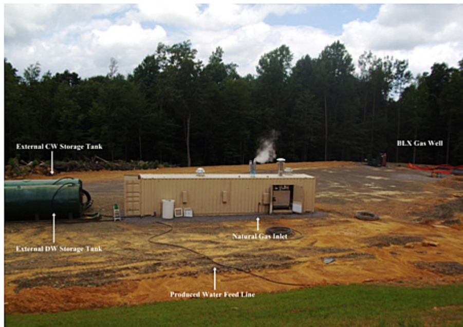
Altela ARS® 4000 system at the demonstration site in Indiana Co., PA.
